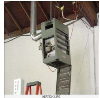
Black stains on the outside of this furnace indicate that pollutants are leaking into the structure.
