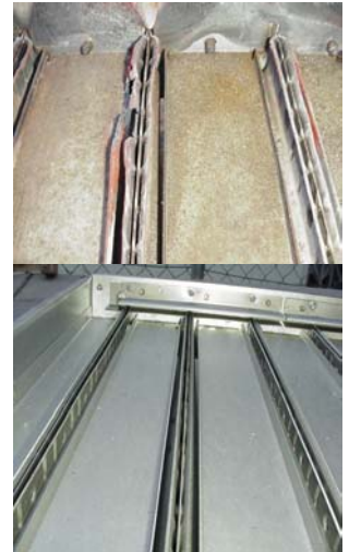
Top- Defective burners. Bottom- New Burners
